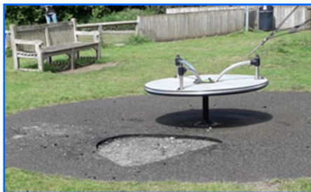
Vandalised flooring at The Willow Centre children's play area
